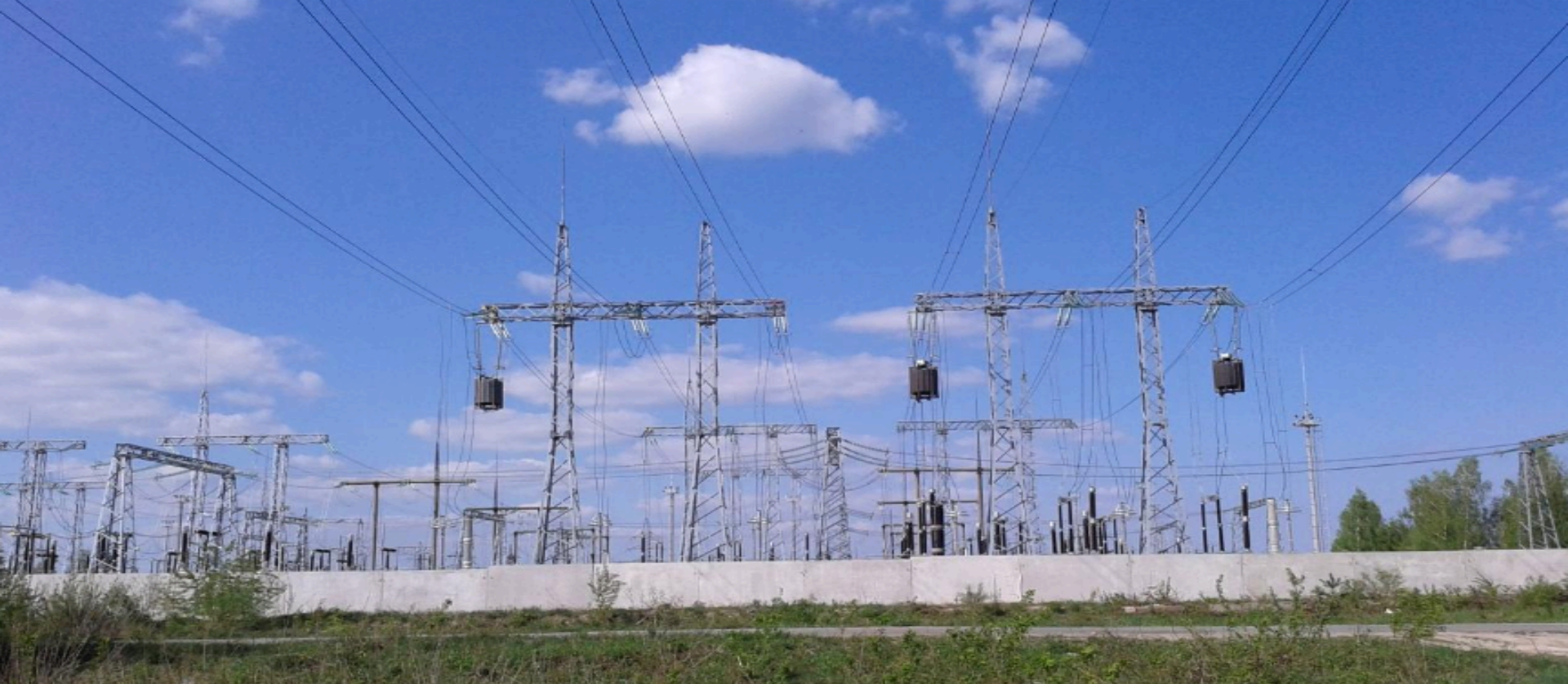
Northern Ukraine Power Grid, North substation in Kiev
